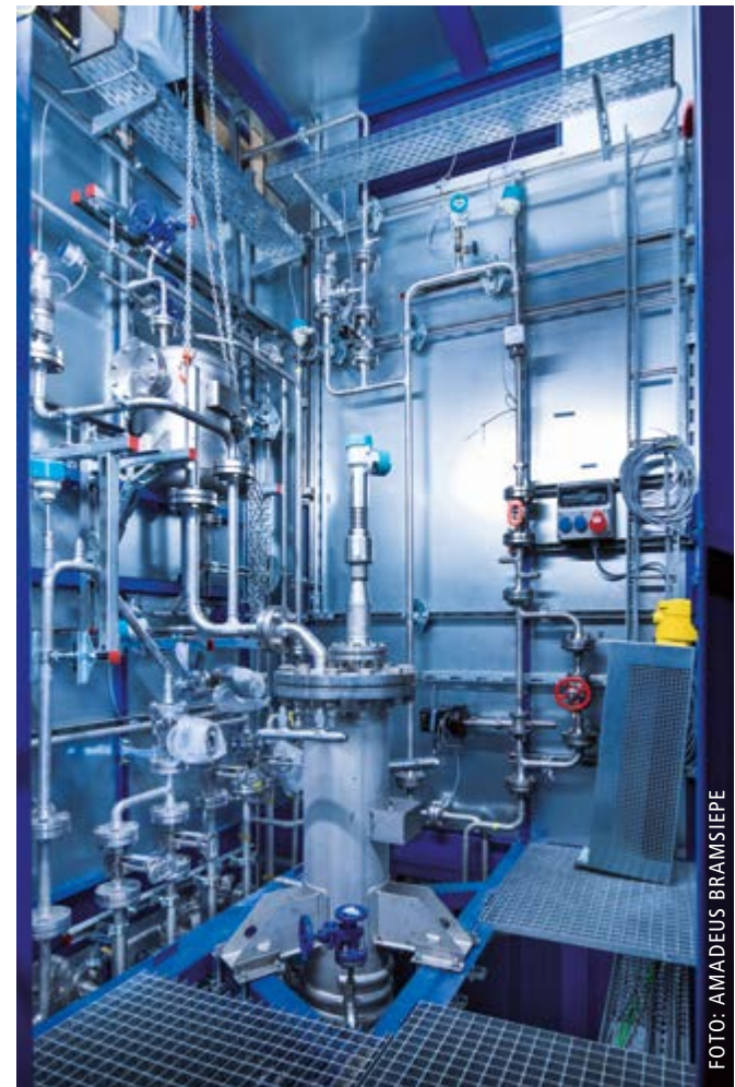
The methanation plant at Energy Lab
