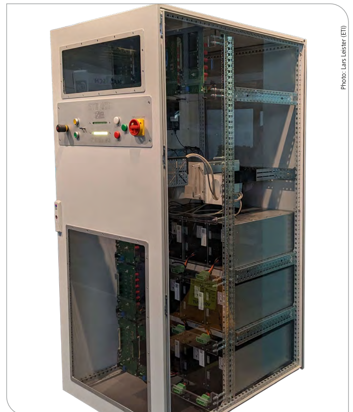
Switch cabinet (arm) - one of the six arms of the overall system.
