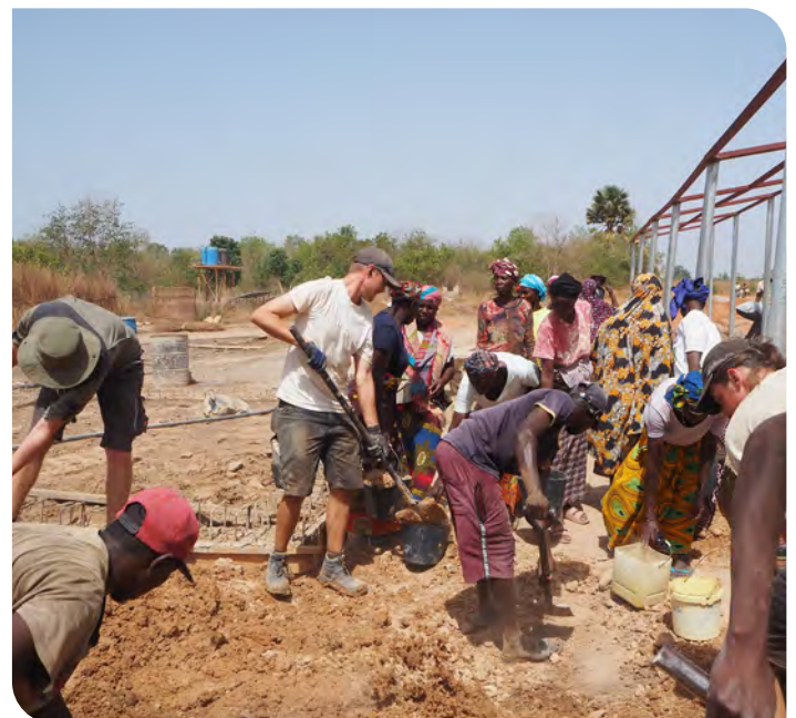
The excavated soil from the toilet pit is used as filling material for the foundations. (EWB, Saba 05/2024)
