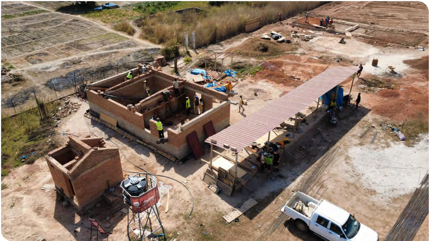
Construction site in Saba: Market area (front right), toilet (front left), meeting and cold storage room (center), and fields (back left). (EWB, 12/2024)
